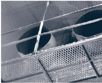
Ice forming on fixtures and equipment, and blocking ducting
